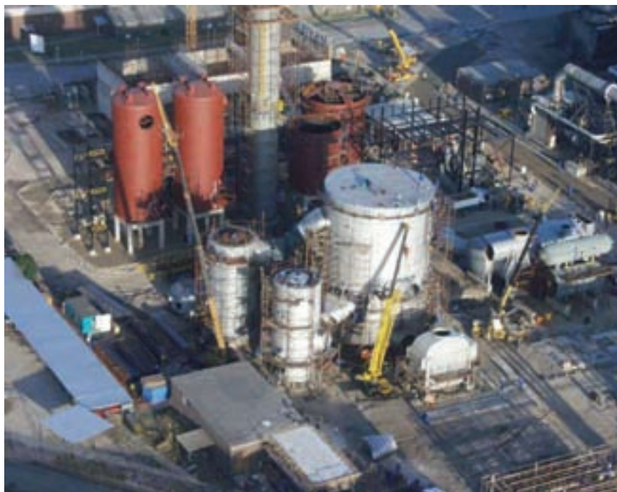
Figure 13 Construction in progress of a new plant to manufacture sulfuric acid at Richard's Bay, South Africa. The construction was completed in 2002 and the plant has the capacity to produce 3,000 tons of sulfuric acid per day.
