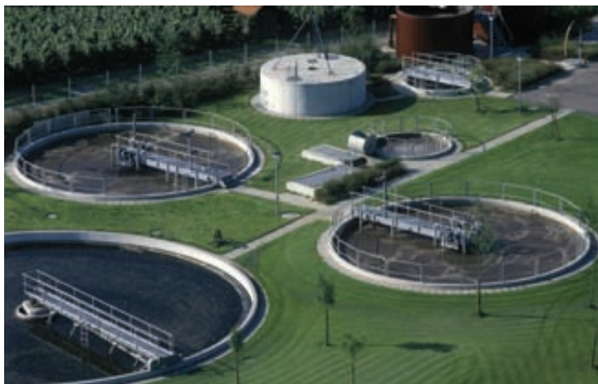
Figure 13 A secondary sewage treatment plant at Shek Wu Hui, Hong Kong
